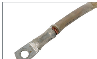
Bare strand protrudes from the broken cable entry.
