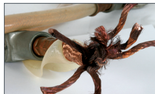
Approx. 30 year old device with a reduced cable cross-section as a result of copper corrosion.
